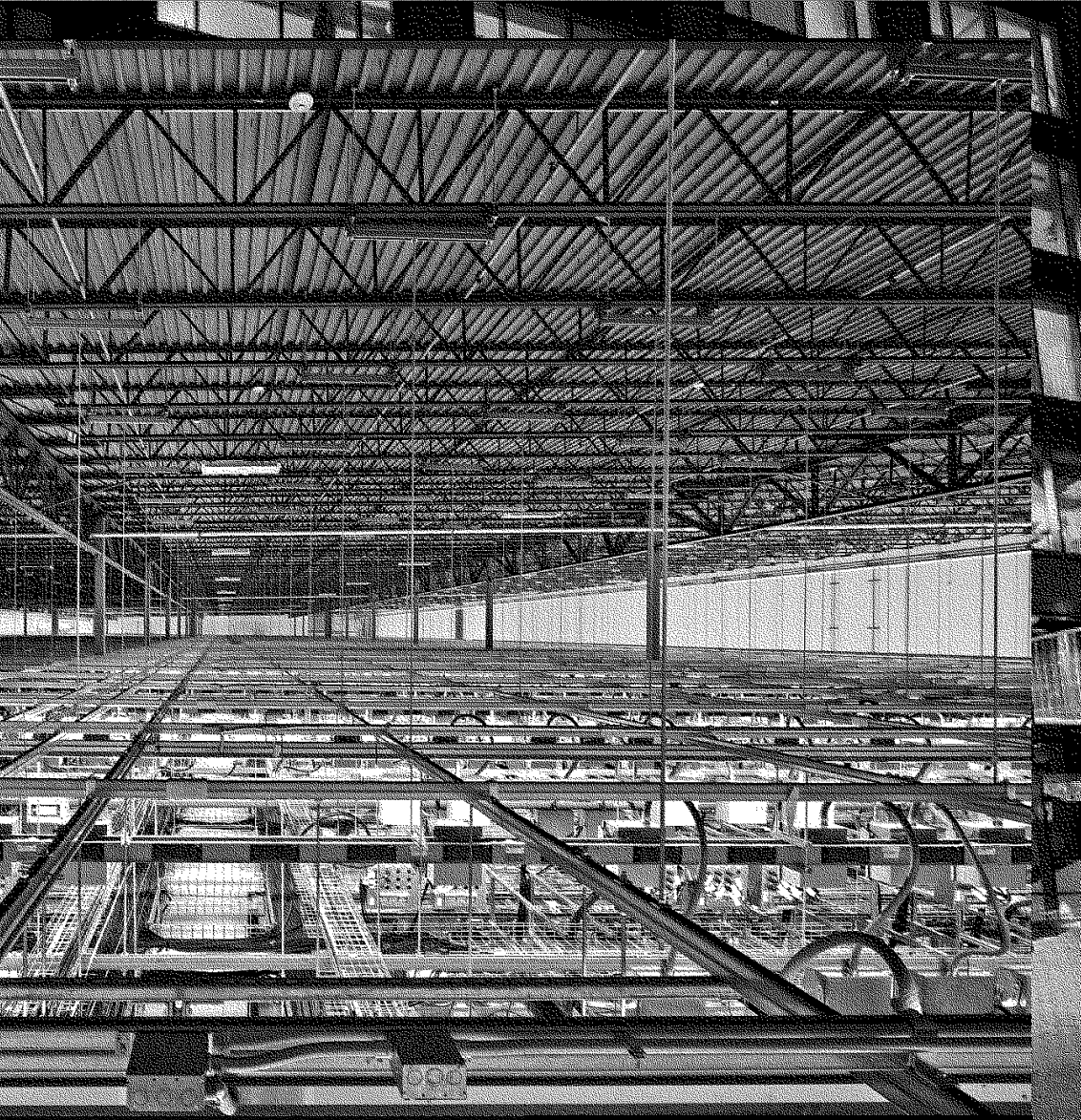
Fig. 5 – Google NC Datacenter, Image (C) Google
